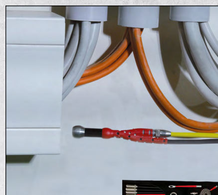
Shafts and underfloor ducting
